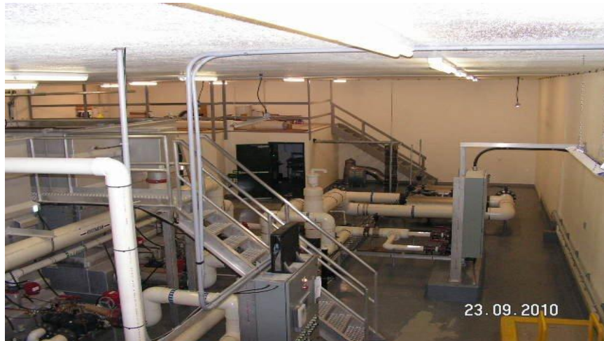
WATER TREATMENT PLANT
