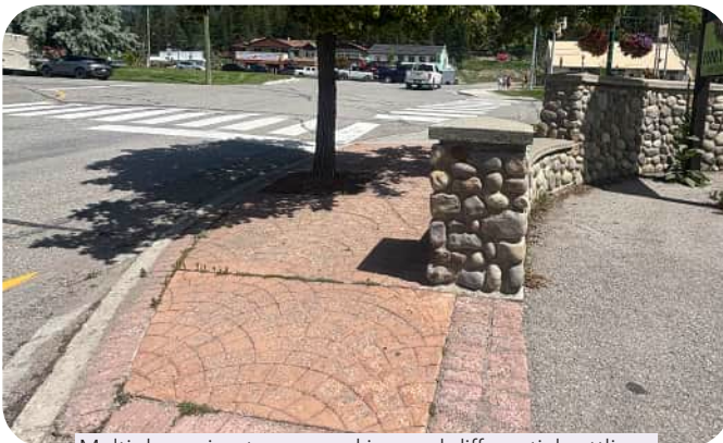
Multiple paving types, cracking and differential settling
