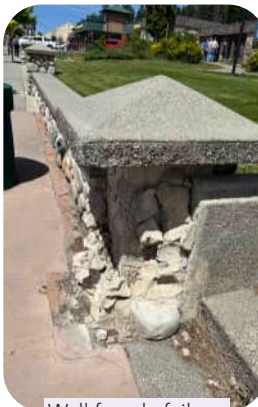
Wall facade failure
